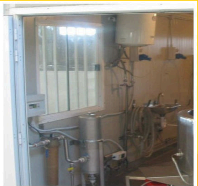
MILK FILTER AND BOILER
